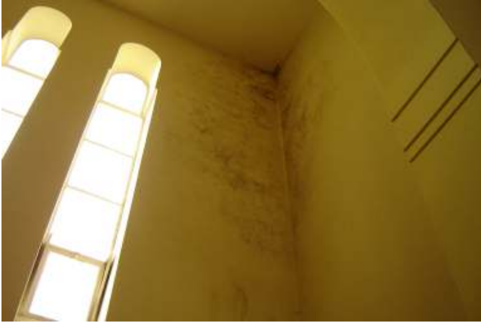
An area of damp on the north west corner of the church.
