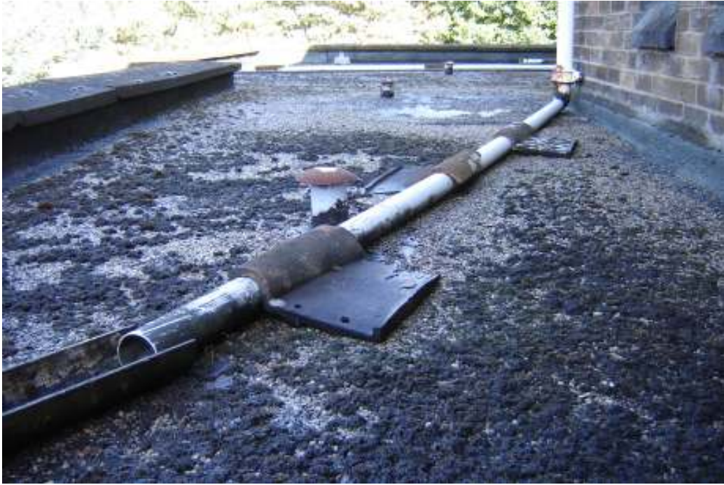
Flat roofs on the west side of the building. Evidence of moss is quite obvious.
