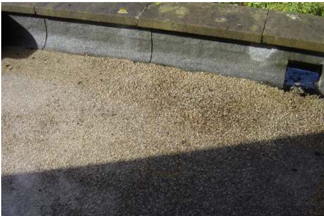
Another shot of that roof. The level of the roof has sunk and is now below the exit for water. As a result the roof is always water logged.
