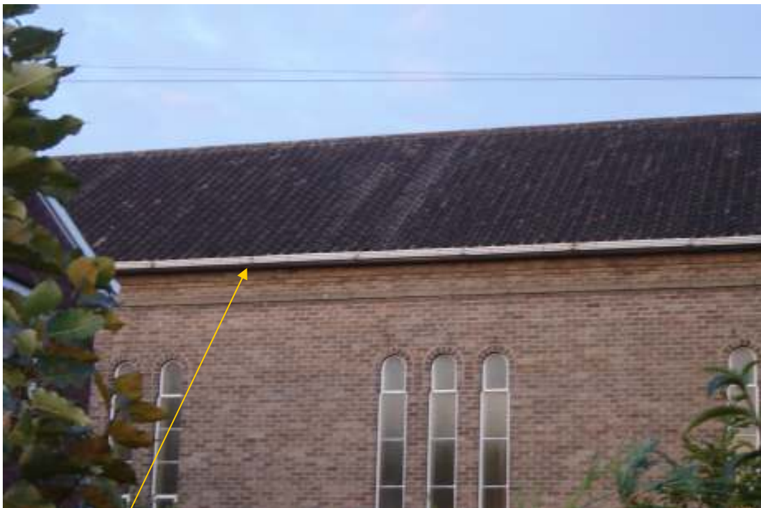
Main roof of the church east side. Signs of corrosion can be seen on the gutters as well as repairing on main roof. The main roof contains no insulation.
