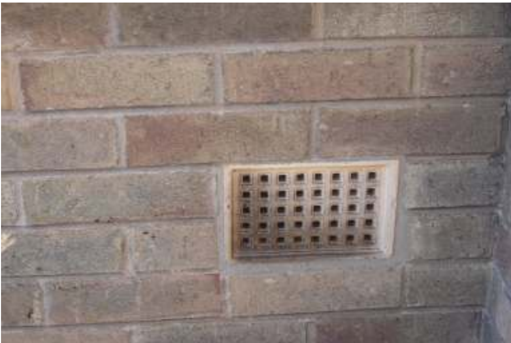
Air grill on the Eastern roof used for nesting by local wasps.
