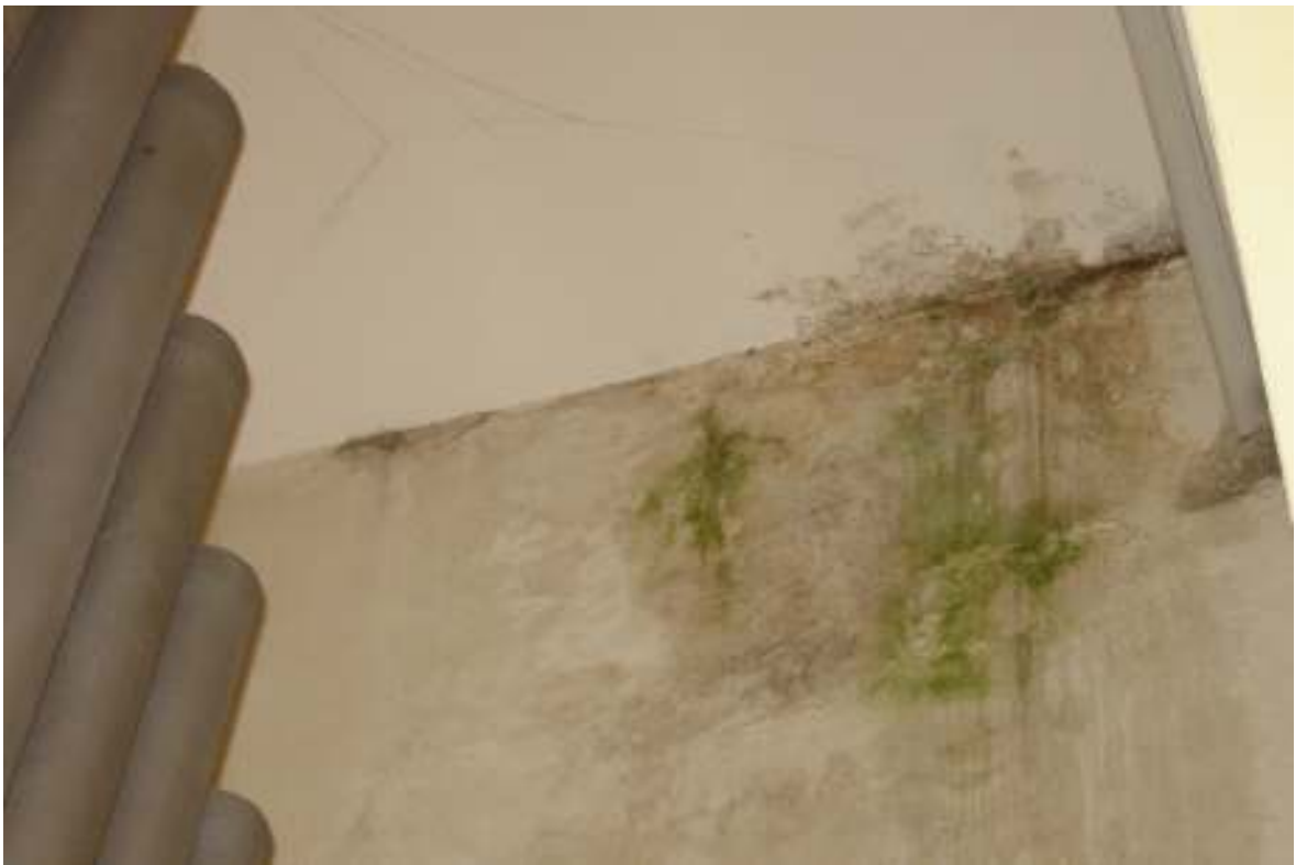
A close up of damp in the choir loft.
