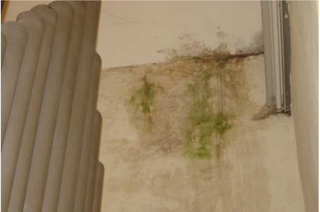
Serious damp problems are in the choir loft. Signs of this damp can also be seen on the outside on photograph 3.
