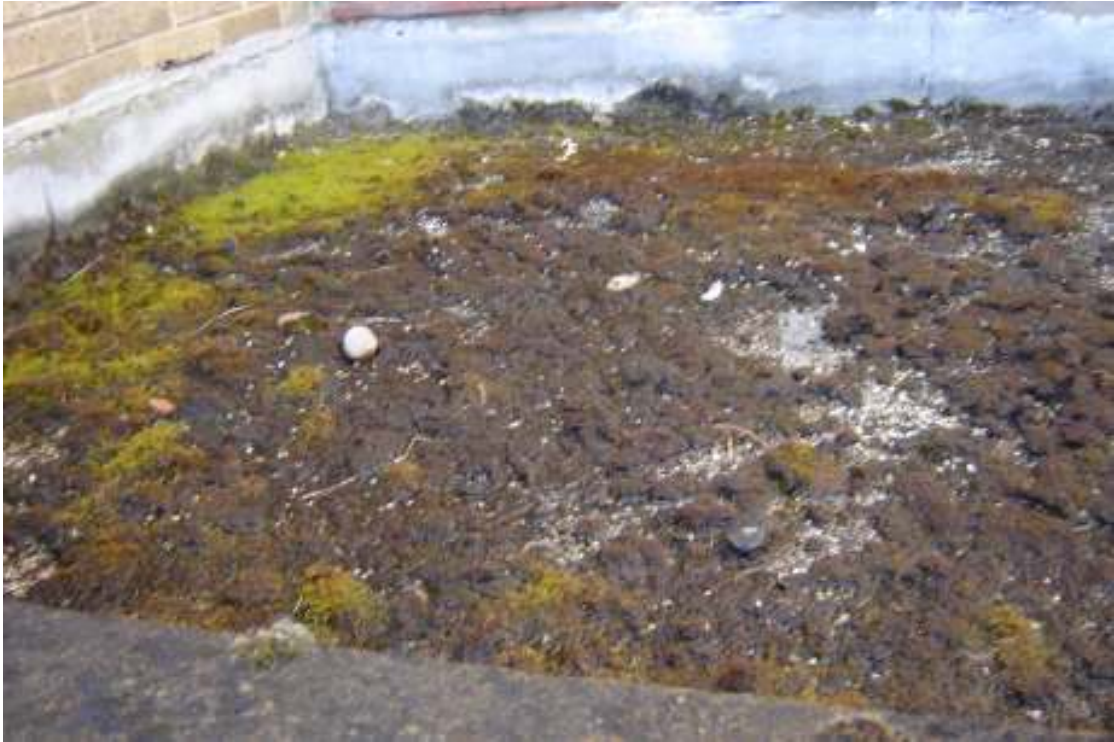
Flat roofs on the east side of the building. Evidence of moss is very obvious.
