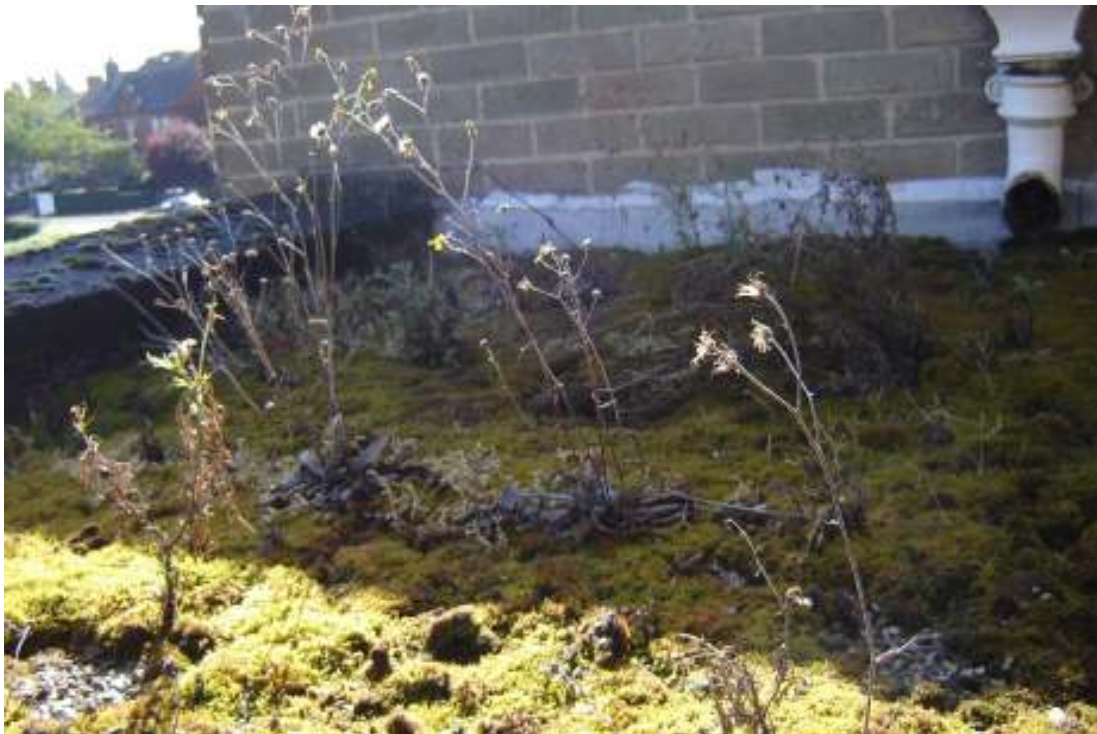
Flat roofs on the east side of the building. A little attention is required.
