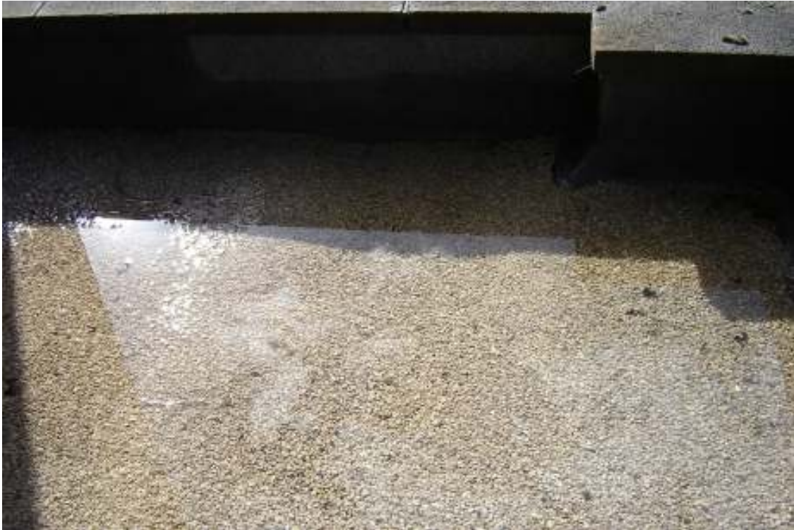
Water lying on the southeast corner of the building unable to drain away.
