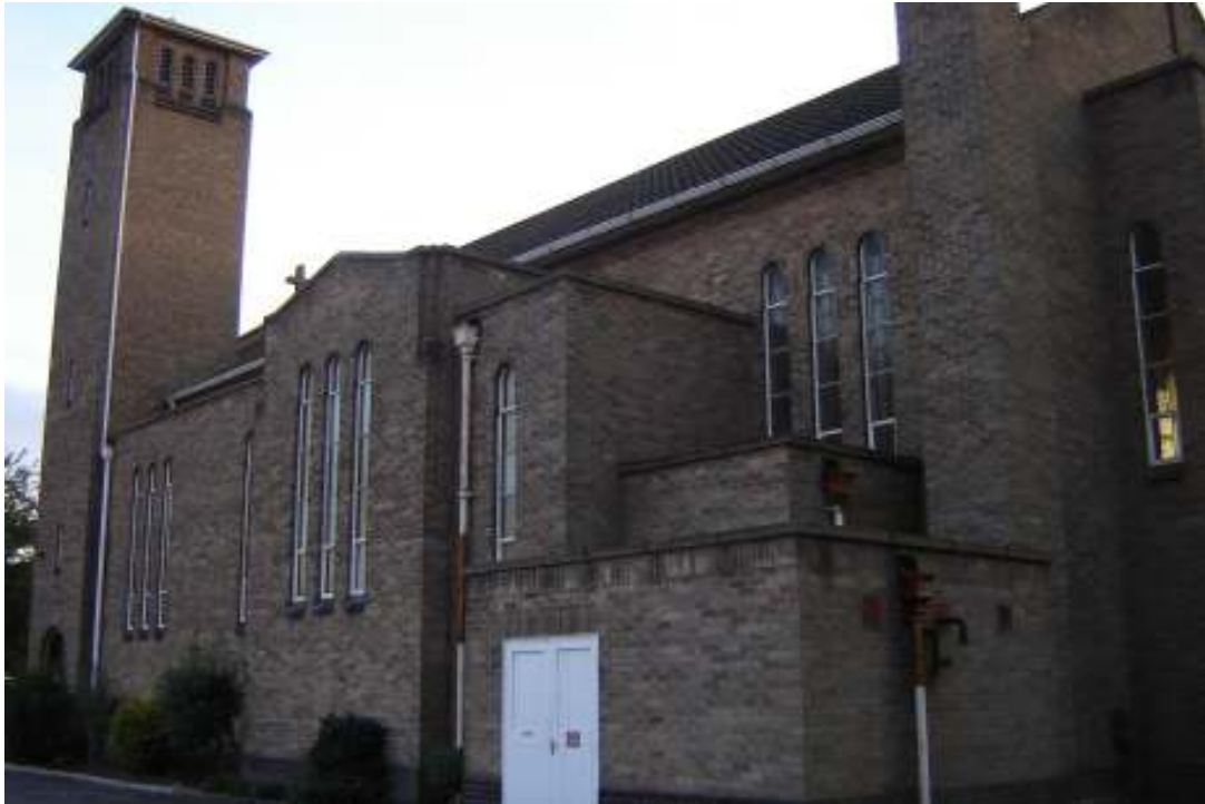
North east corner of the church showing flat roofs and church tower. Water pours over the top of the tower.
