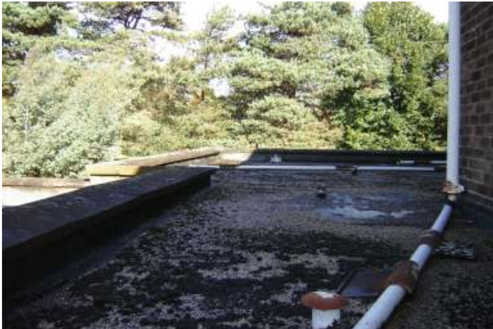
Flat roofs on the west side of the building. There is evidence of bubbling and cracking.
