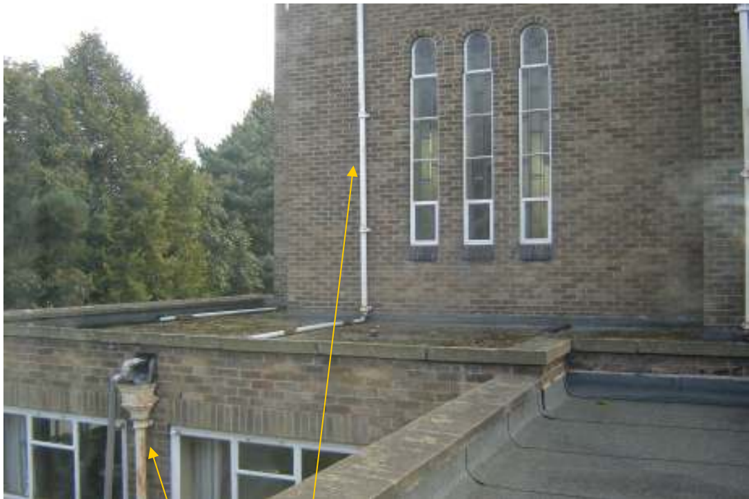
Flat roof north west corner of the church. Notice conditions of downspouts.
