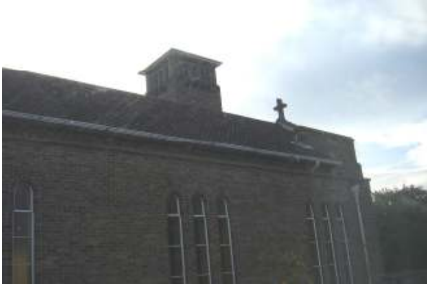
Another shot of the west side of church. Rainwater goods need to be replaced.
